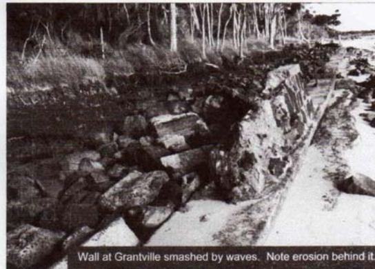
Wall at Grantville smashed by waves. Note erosion behind it.
